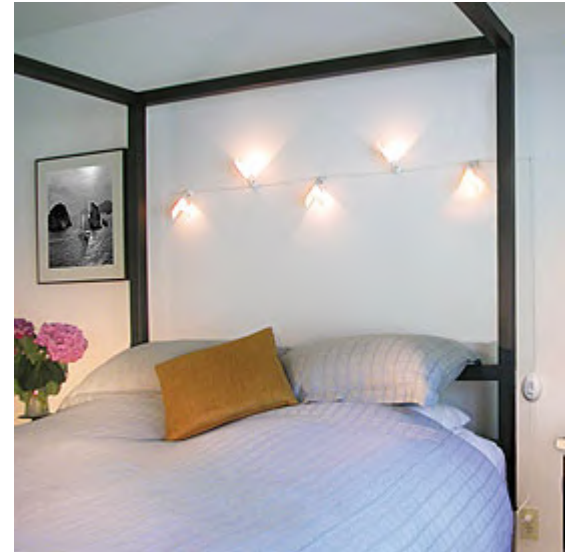
Halogen Track Lighting
