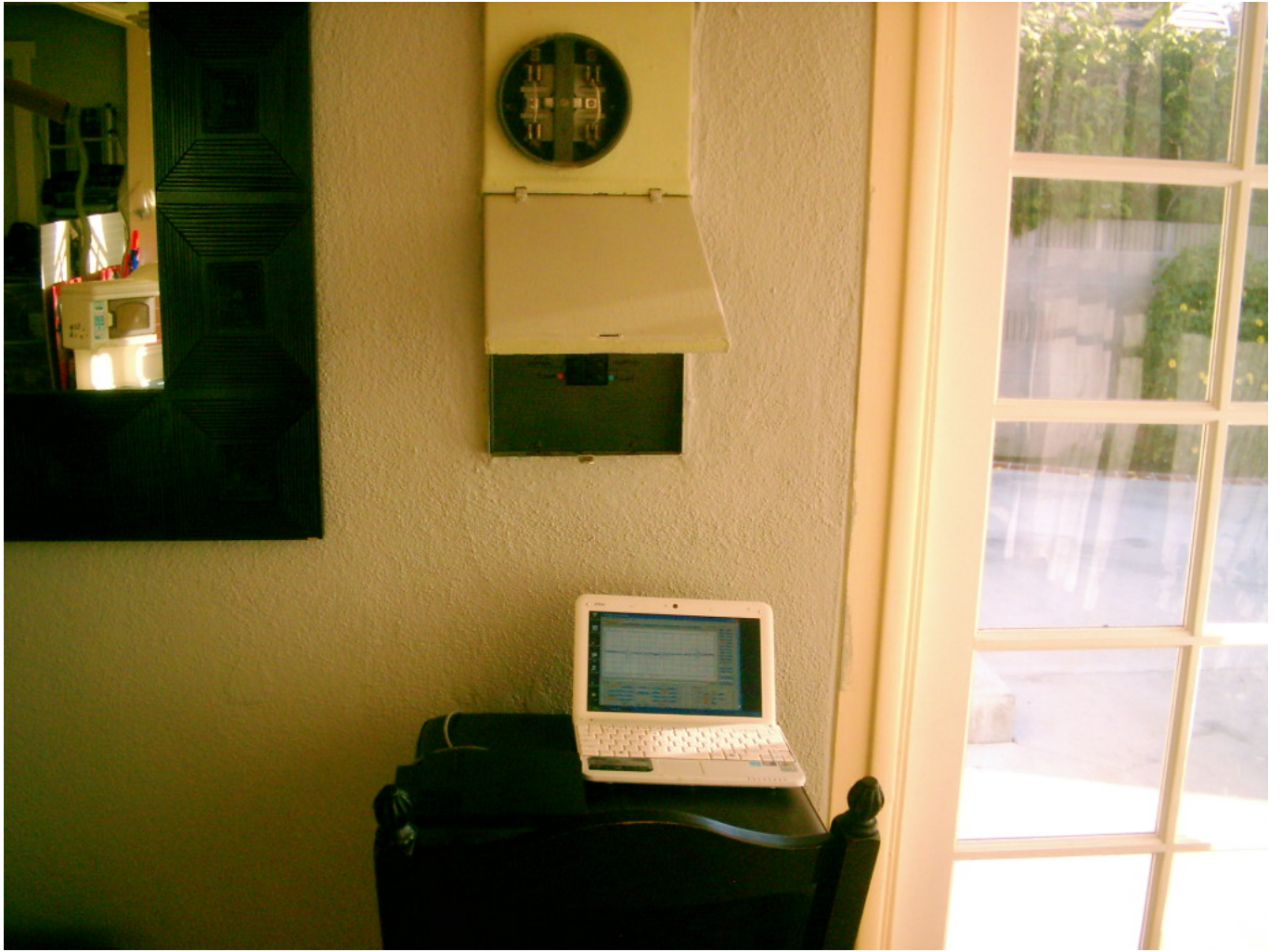
Here is the oscilloscope held next to the empty meter base, showing the presence of the voltage harmonics even with the smart meter removed:
